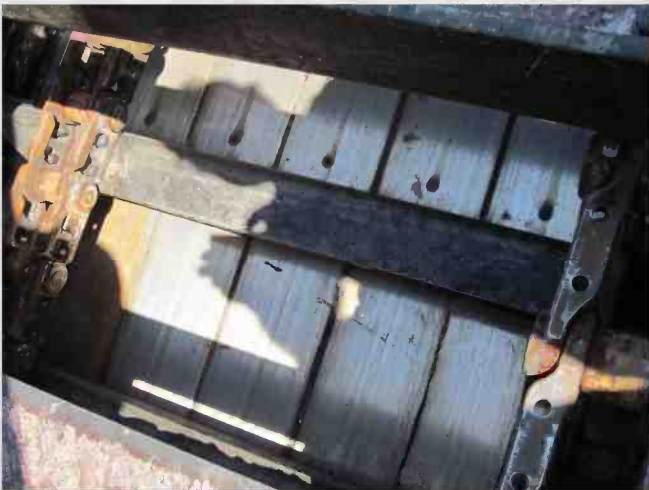
Kenco Perma-Liner floors in pickup machine
